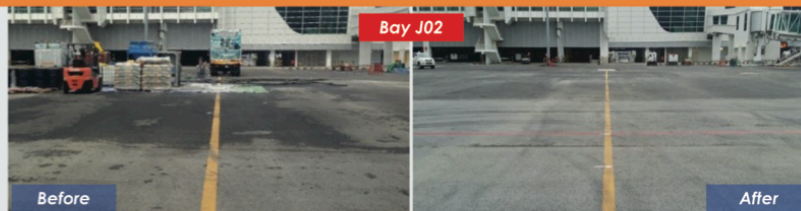
Bay J02 free from water ponding after the completion of grouting injection works.
